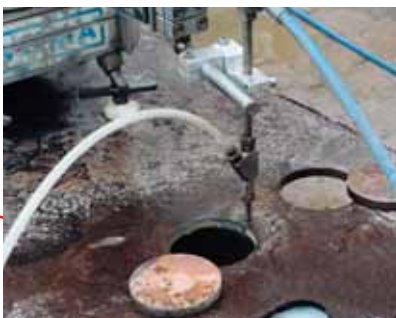
On-site cutting of openings in walls and ceilings with the 3000-bar circular abrasive cutter Eco Top Cutter.
