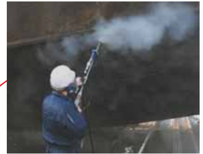
Weld seam cleaning and scale removal with the 3000-bar Modular Gun System.
